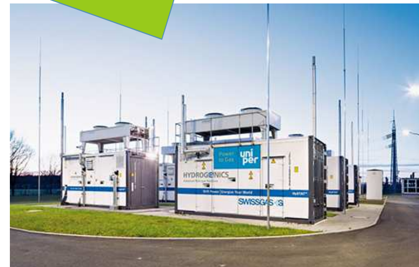
Existing electrolysis systems at Falkenhagen © Uniper Energy Storage GmbH
